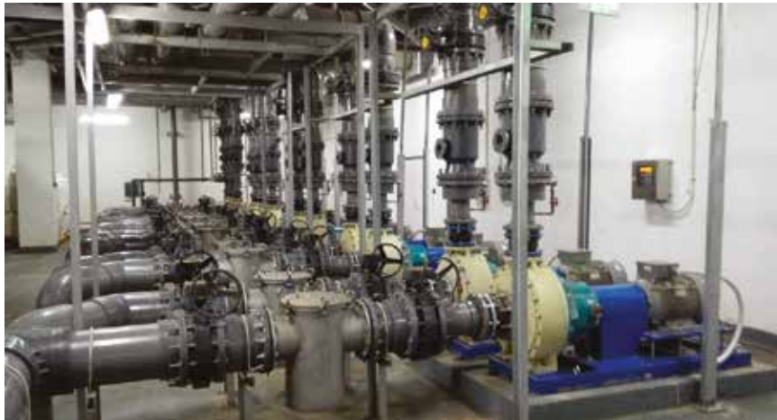
CHINA, Aquatic Park - Supplying tank with sea water
