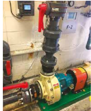
USA, Chemical plant - Caustic soda transfer
