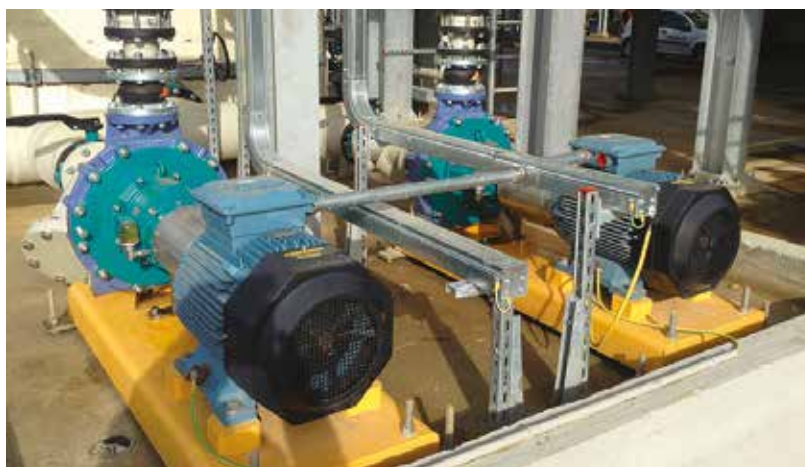
ITALY, Desalination plant
