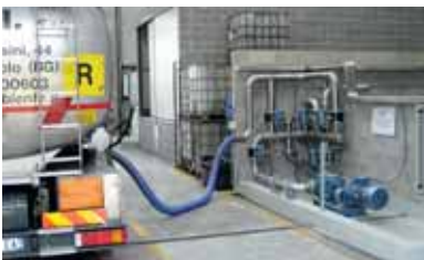
RECOVERY OILS PLANT
