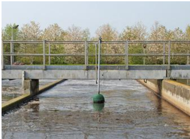
Oxix ® Ball Float solution fitted to a railing in a water treatment facility.
